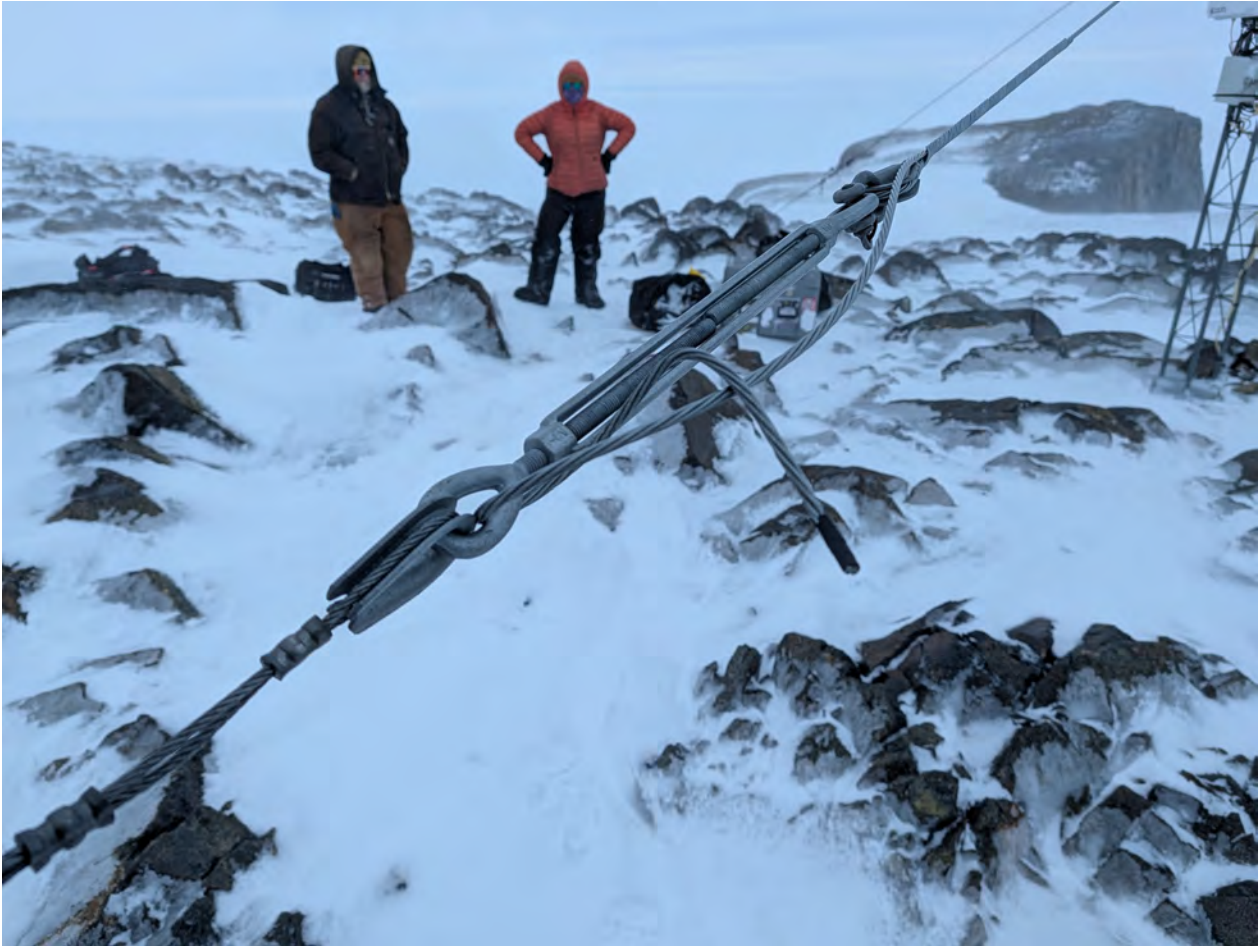
Turnbuckle assembly for tower rigging
