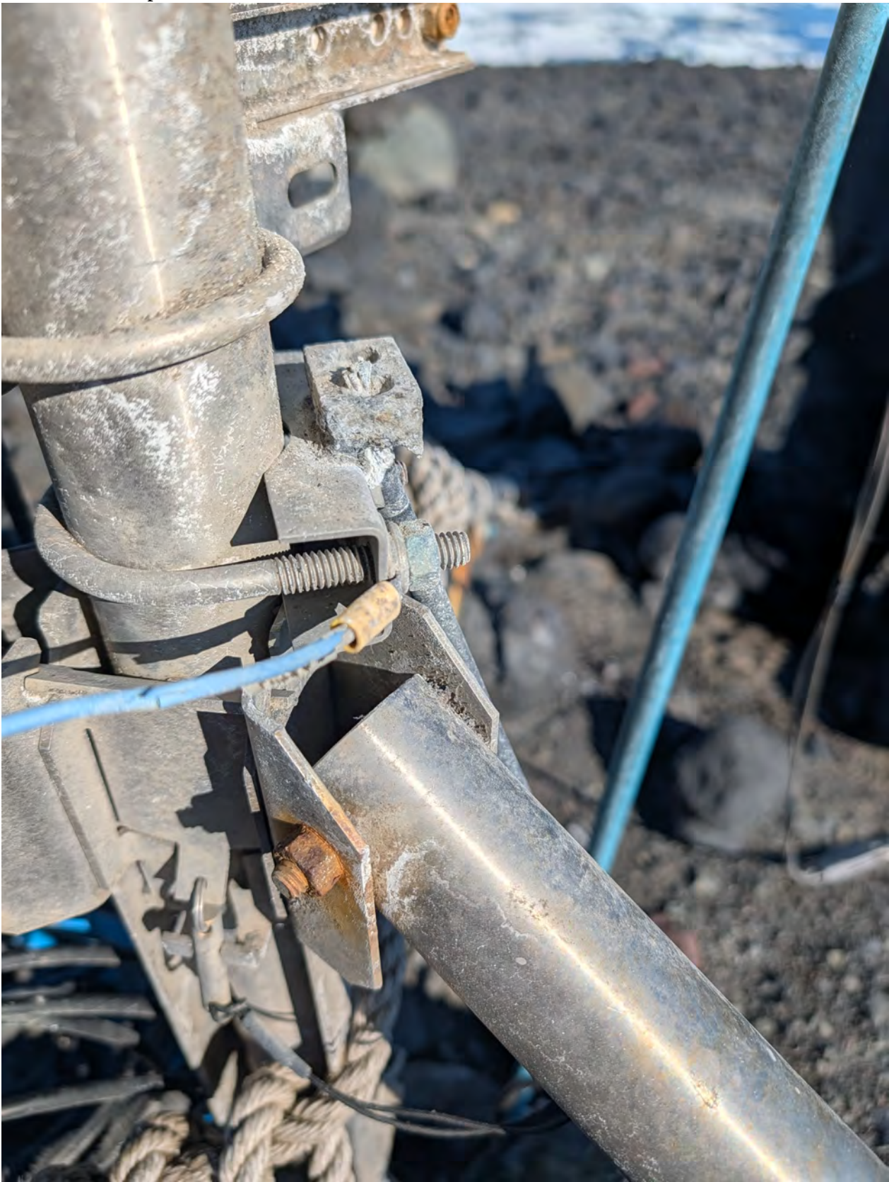
Light corrosion on tripod hardware
