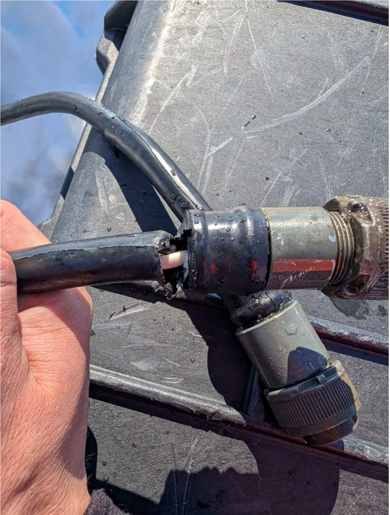
Power system cable strain reliefs - cracked
