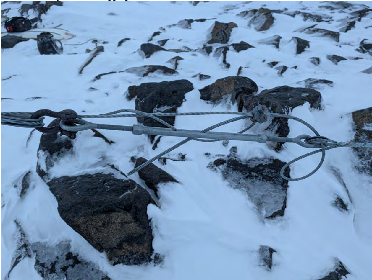
Turnbuckle assembly for tower rigging
