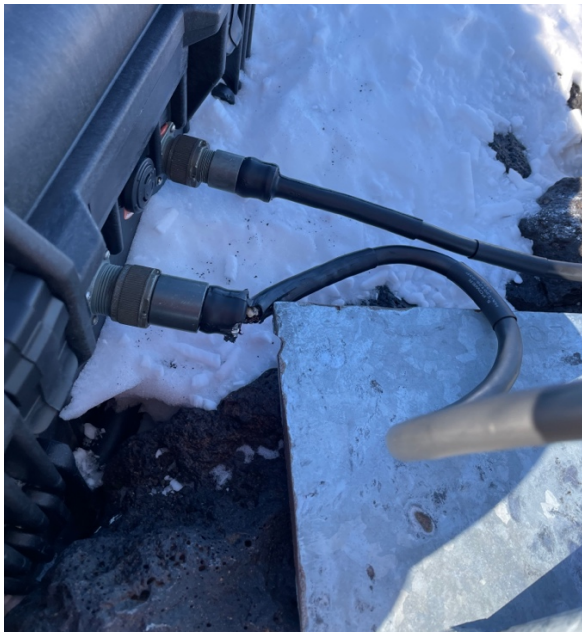
Upon arrival, noticed damage to power cable.
