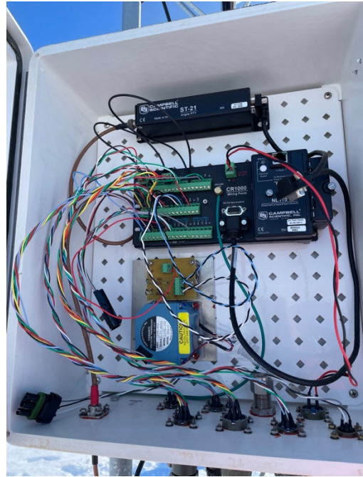
Inside GIL enclosure.
