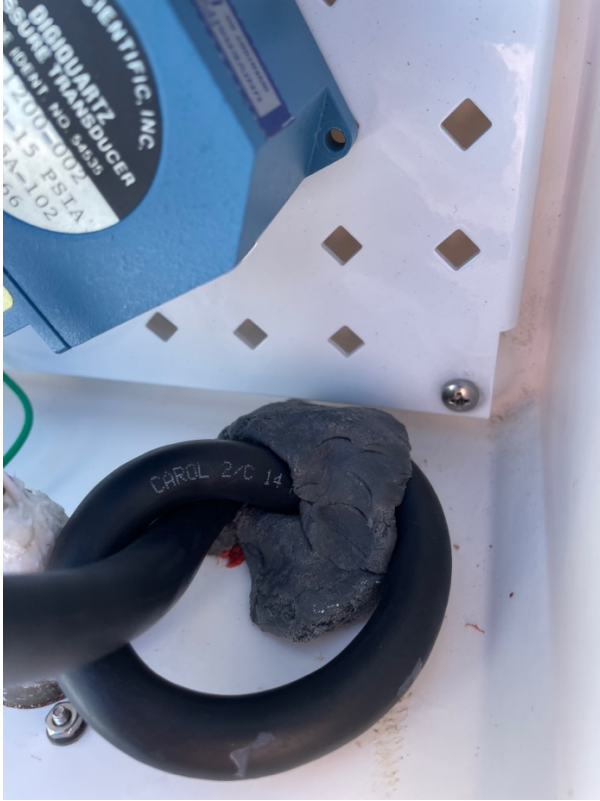
Power cable w/ putty, inside enclosure.
