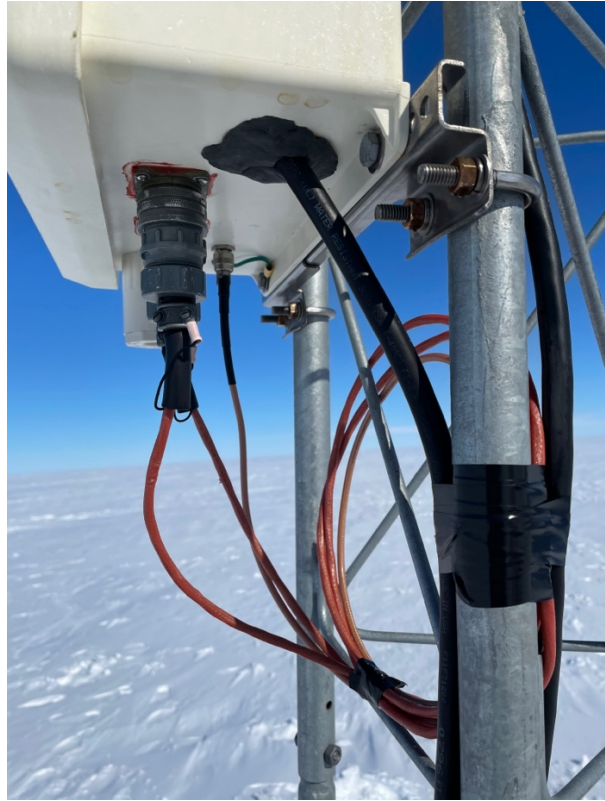
Bottom of enclosure.
