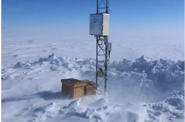
Batteries now under enclosure.
