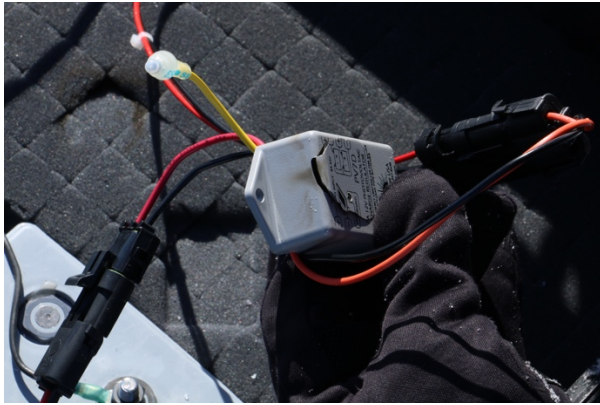
The damaged charge controller.
