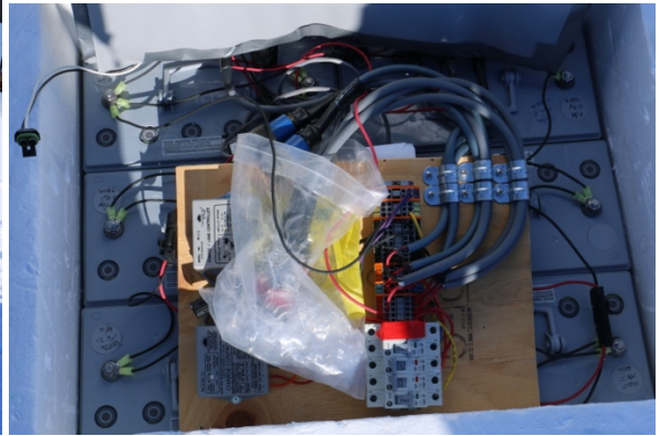
Inside the power system.
