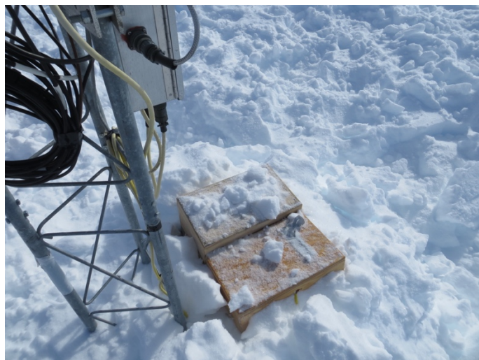
Battery boxes. Note power cable coming out of box.
