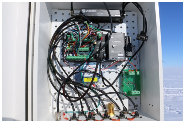
Inside ELZ enclosure.
