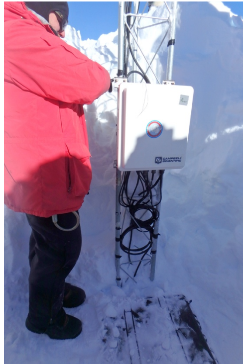
The new power system.
