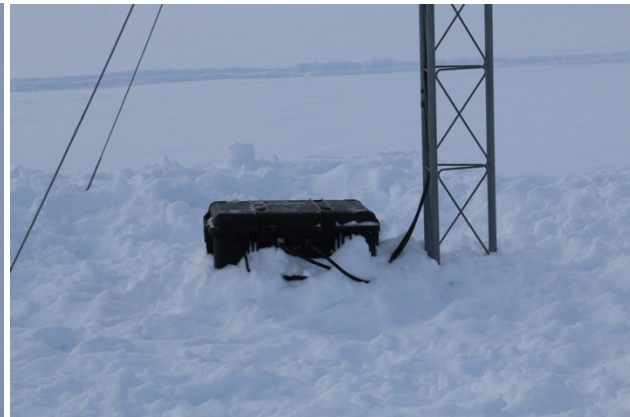
The power system.
